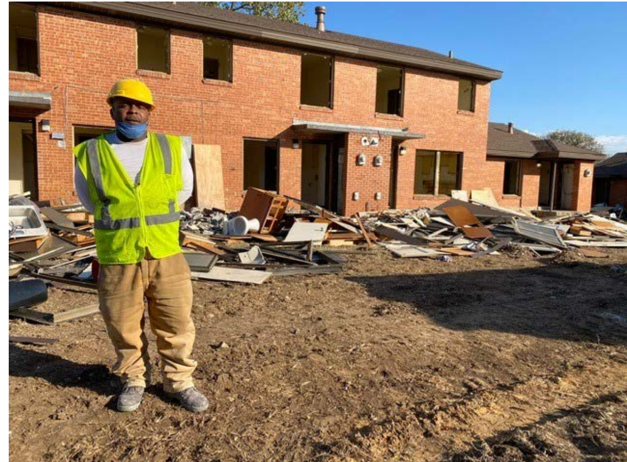
Mark Anderson grew up in Cavile Place and was hired in Fall 2020 to assist with demolition work through HUD's Section 3 program.
